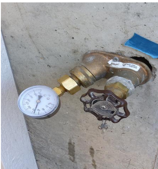
Photo to show the water pressure gauge reading approximately 72 psi.
