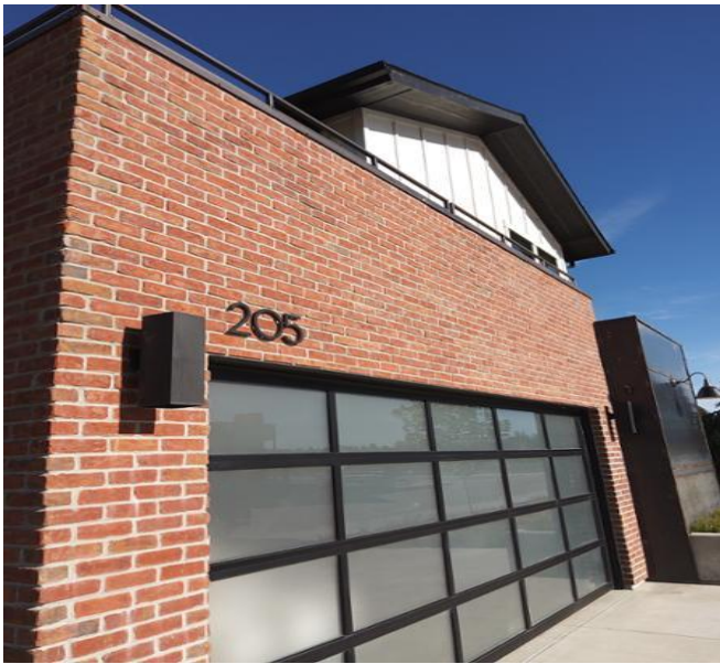
Photo to show example of the brick siding at the 2-car garage.
