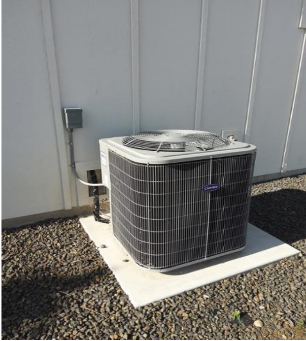
Photo of the exterior A/C unit.
