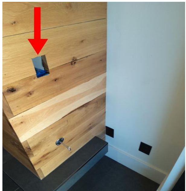
Photo to show the open junction box at right of fireplace.
