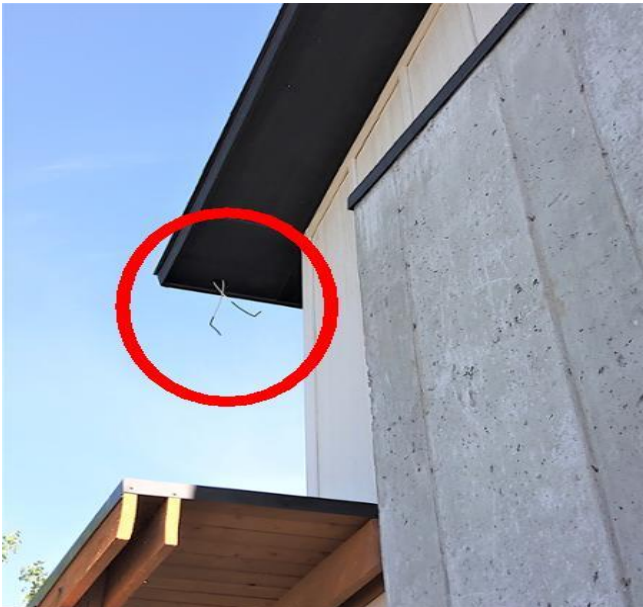
Photo of show the observed exposed wires hanging. Suggest repair.
