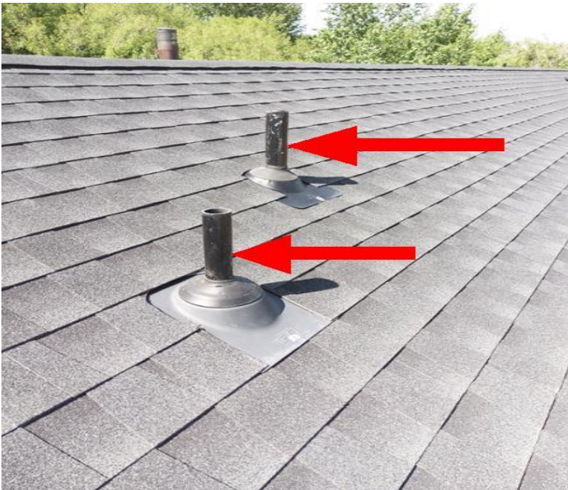
Example of the plumbing vents.
