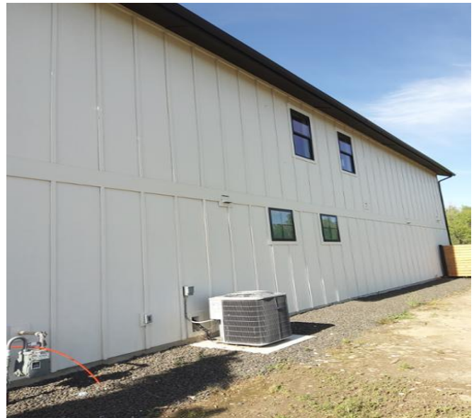
Photo to show the siding at the north side of the garage and house.
