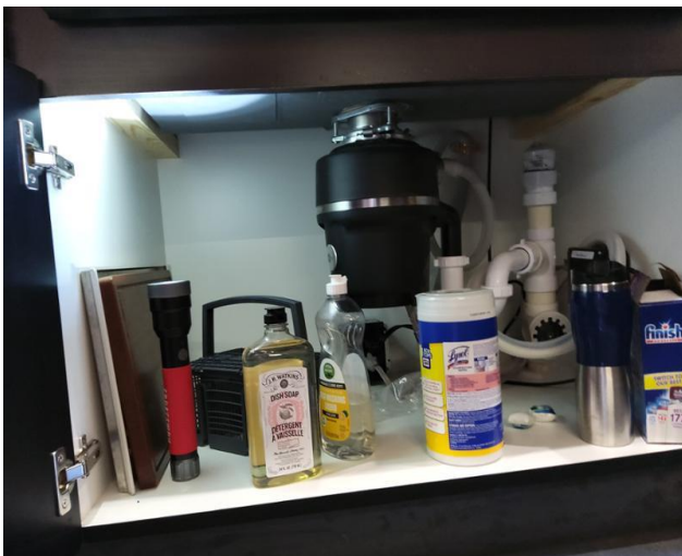
Photo to show the Kitchen sink plumbing.
