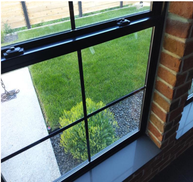
Photo to show example of the missing window screens at dining room.
