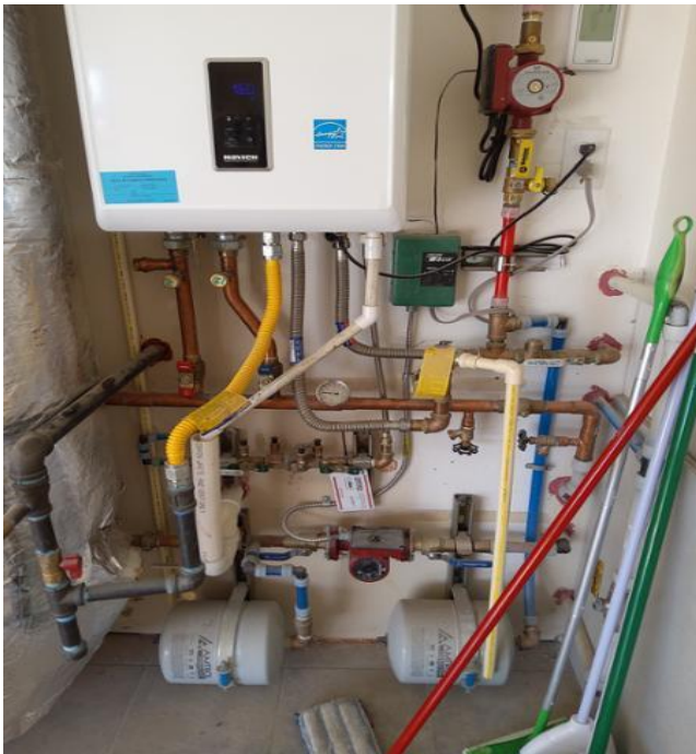
Photo to show the water heater and heated floors components.
