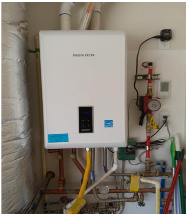
Photo of the tankless water heater system.
