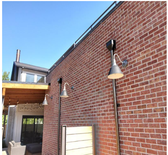
Example of the masonry siding at the south side of the house.
