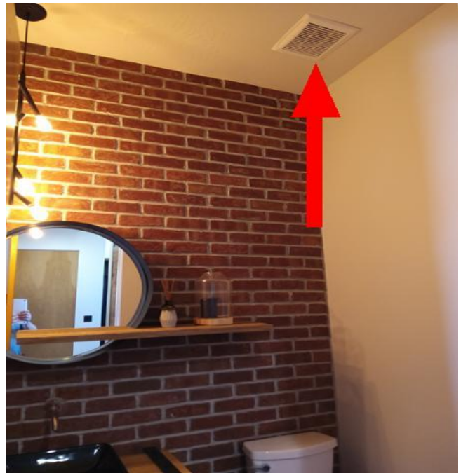
Photo to show the location of the exhaust fan. Did not work at time of inspection.
