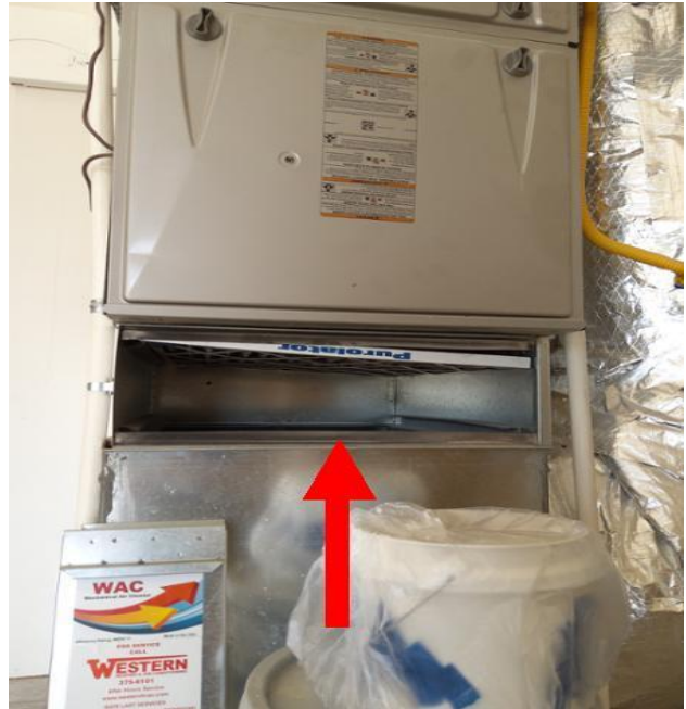
Photo to show the appearance of incorrect furnace filter installed.
