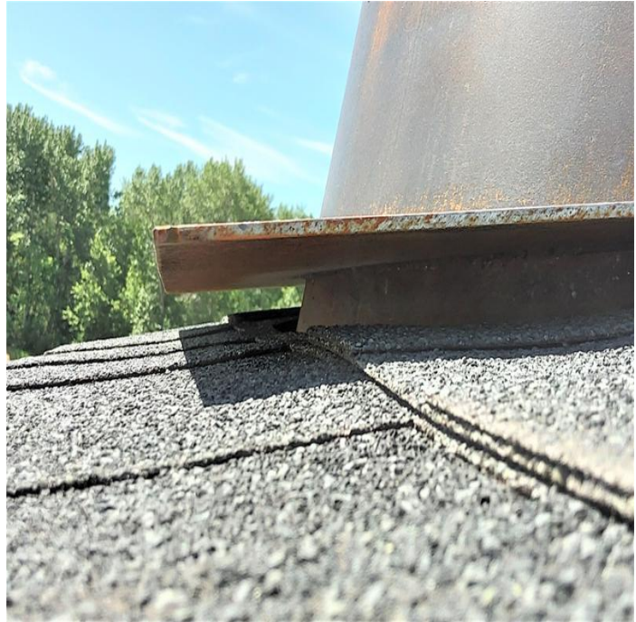
Photo to show the observed gap at chimney flashing. Suggest repair.
