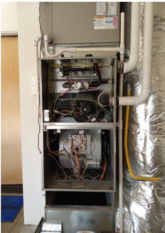
View of the furnace with cabinet cover removed.
