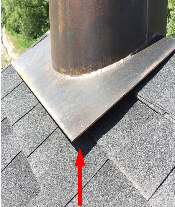
Photo to show location of the observed gap at flashing.
