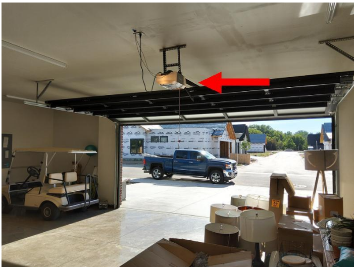
Photo to show the garage door opener.
