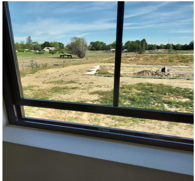
Observed missing window screen.
