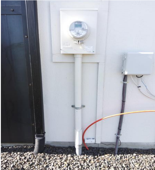
Photo to show the electrical service entry for the house.
